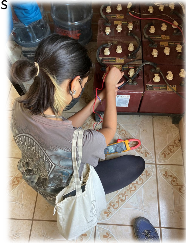
Joya Debi (EE '23) measuring batteries
